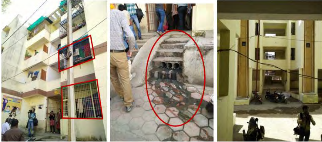
Fig. (15) and (16), Bhopal Rahul Nagar project under BSUP schema, Fig. (17) Ambedkar Nagar Project under BSUP schema, Bhopal Source: Photos by the author
