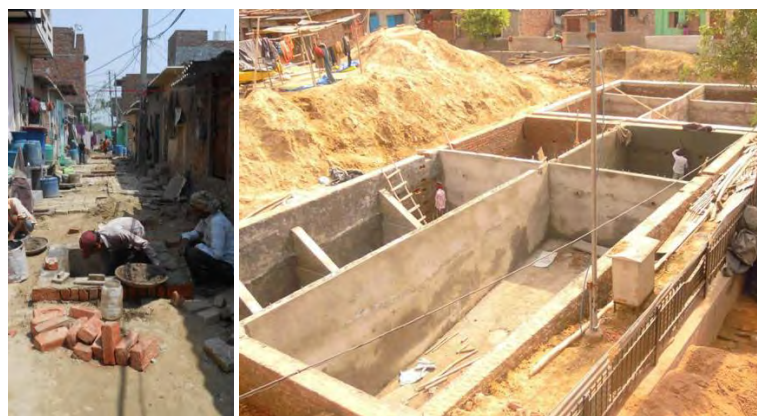
Fig. (24) and (25), Delhi, Savda Ghevra, Cluster Septic Tank and Simplified Sewer for Home Toilets Source: (CUREINDIA, 2016)
