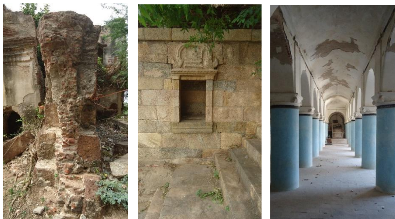
Figure 3: Section of a three-leaf masonry wall at Vennar Chatram showing the two layers of laterite and a center brick layer with lime mortar (left); the steps leading to the Vennar river at Vennar Chatram made up of sand stone (center); interior of Kalyana Mahal finished with lime plaster (right). (made by the author)
