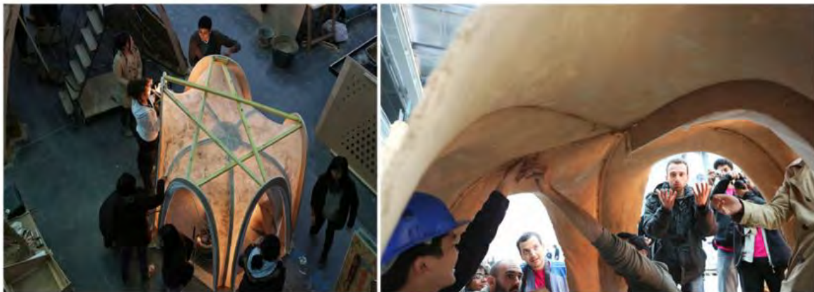
Figure 3. (a) First layers of claymix applied by hand by more than 3 people working simultaneously. (b) Removal of the wooden arches and fabric formwork.
