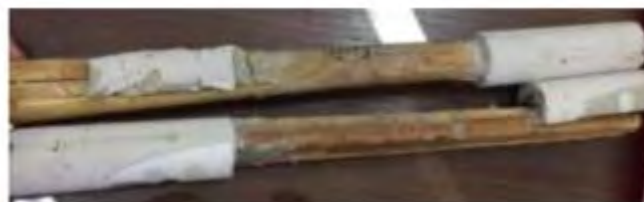
Figure 20. Zoom in on the longitudinal cracks under the Epoxy (Author's own, n.d.)
